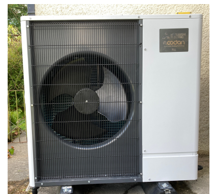
Air Source Heat Pump
